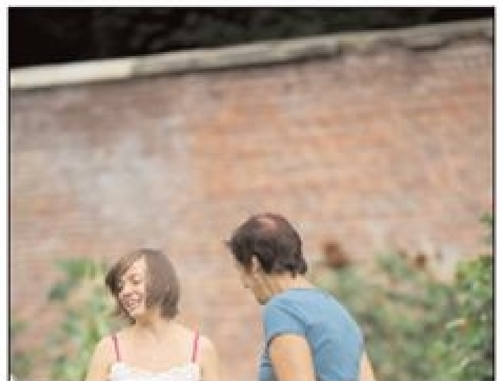
Daniella (left) with Chris M. Note the new section of specially made moulded coping stones replaced by Booker & Best (commissioned by HBC). Without the coping stones, the wall quickly becomes damaged through rain.
